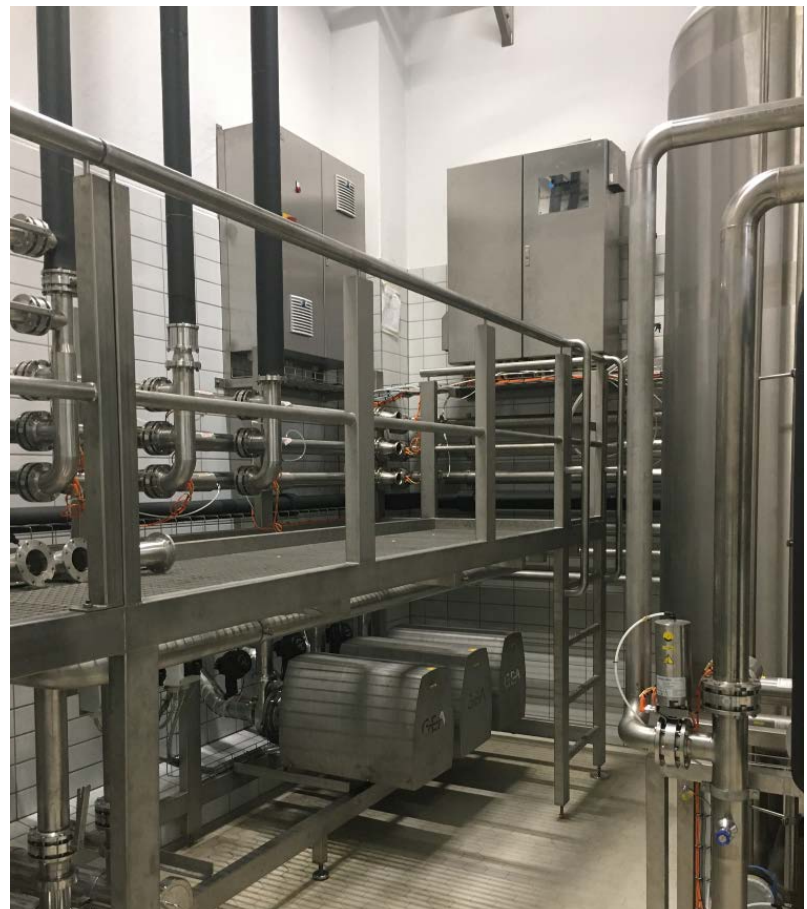
Mineral water supply with distribution manifold
